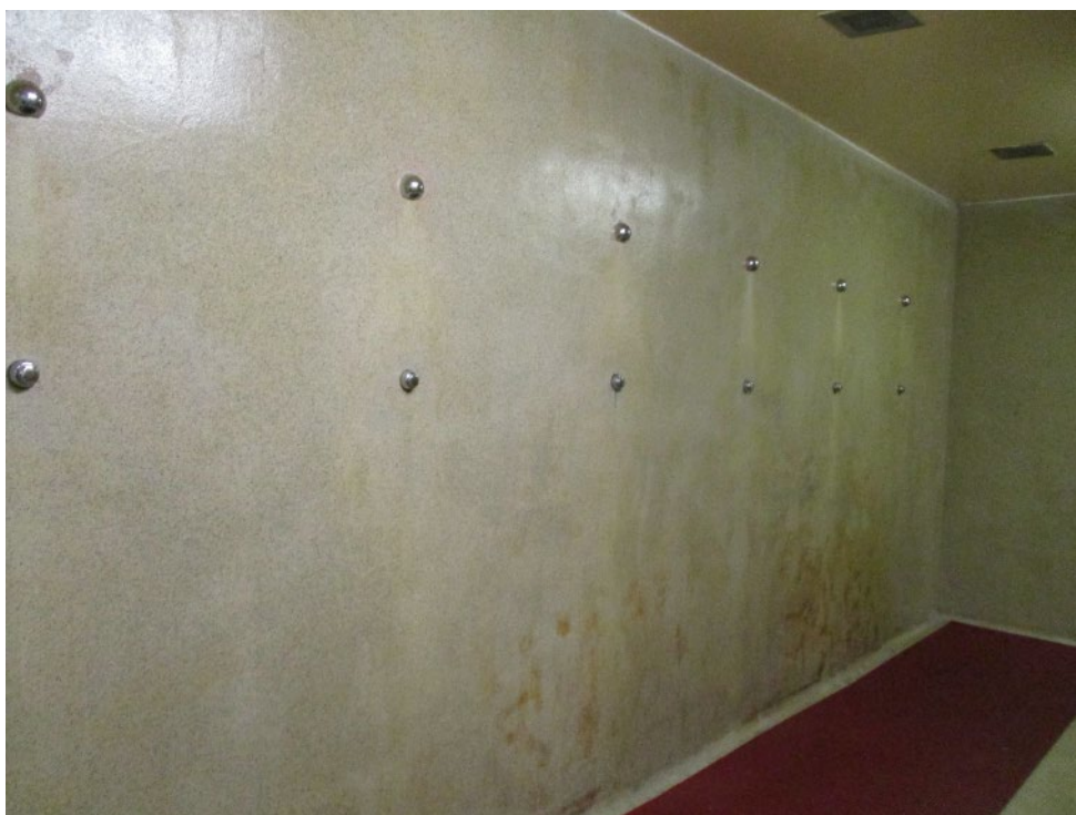
Gym showers in need of refurbishment
