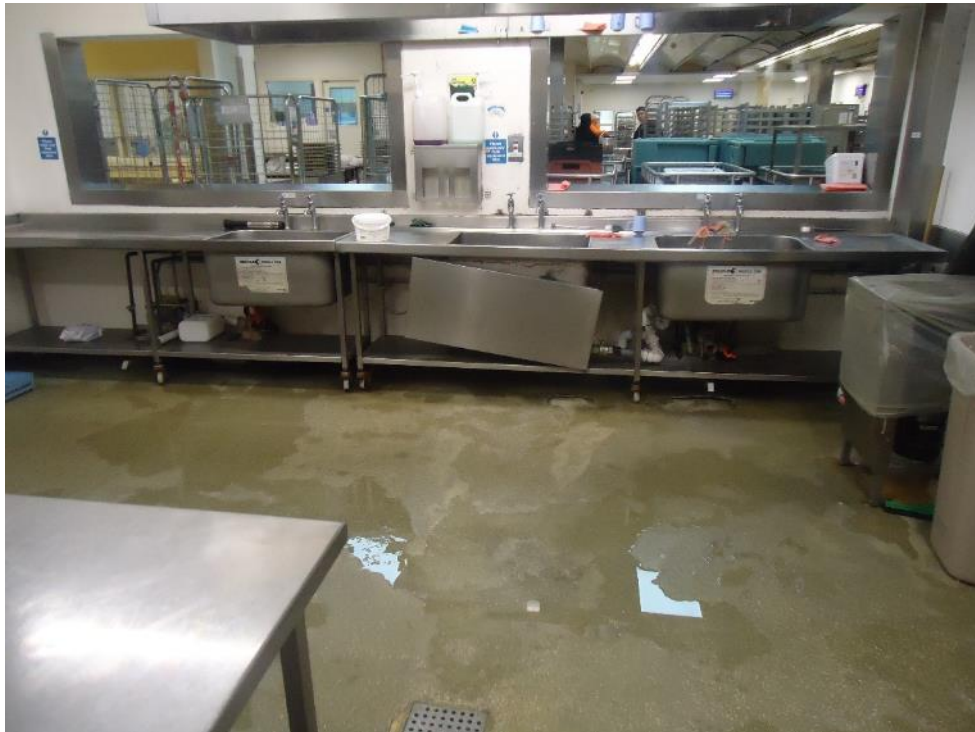
Broken sinks in kitchen
