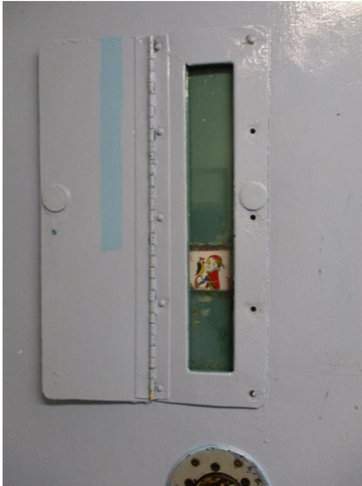
Obstructed observation panel
