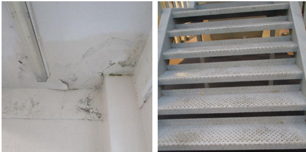
Mould in the D wing association room (left) and ingrained dirt on F wing stairs
