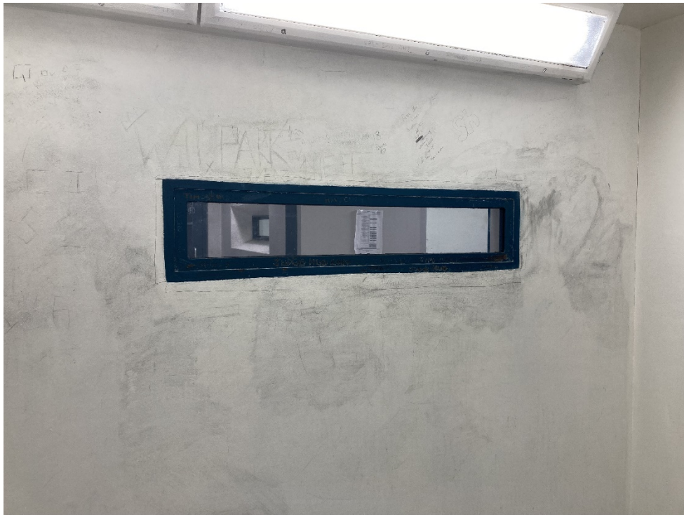
Dirty cell wall at Doncaster Crown court
