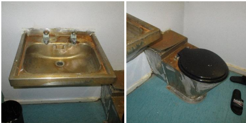
Rusty sink and filthy toilet in segregation unit cell
