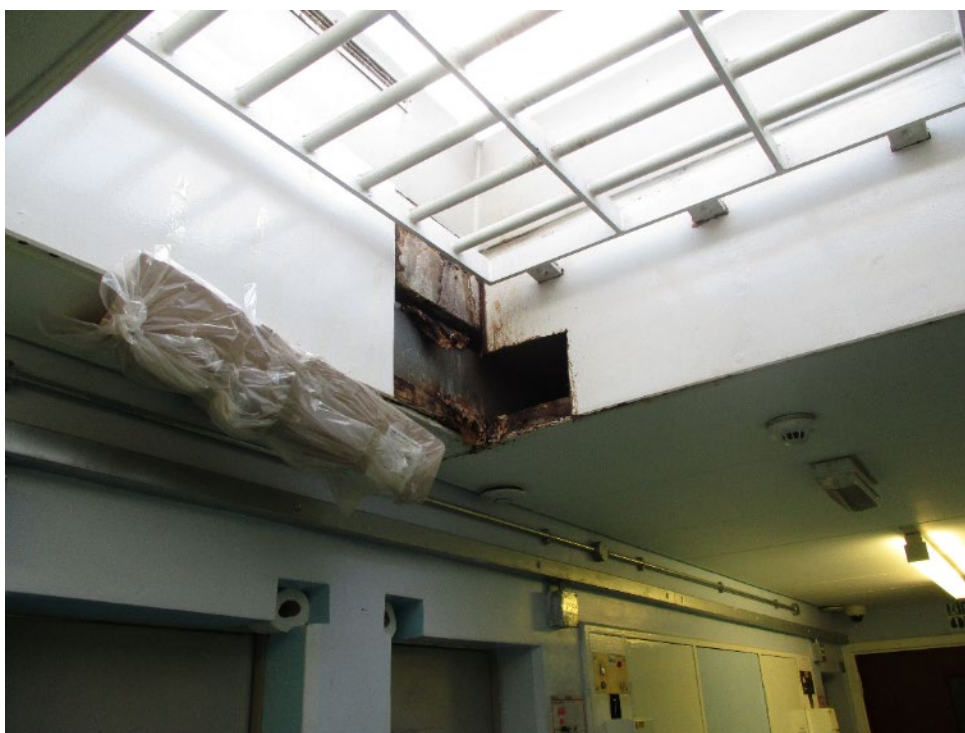
Leaking roof in segregation unit
