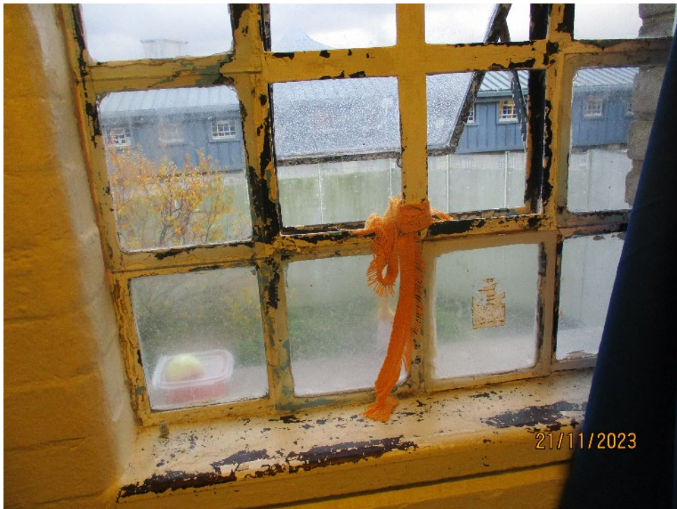
Damaged window frame
