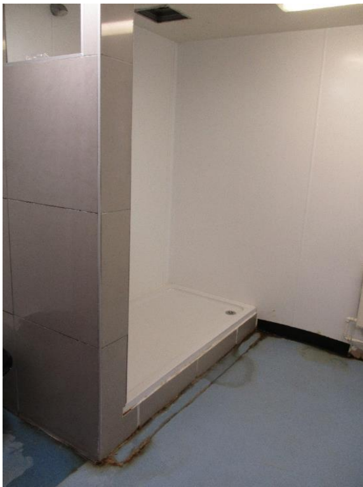
Segregation unit shower
