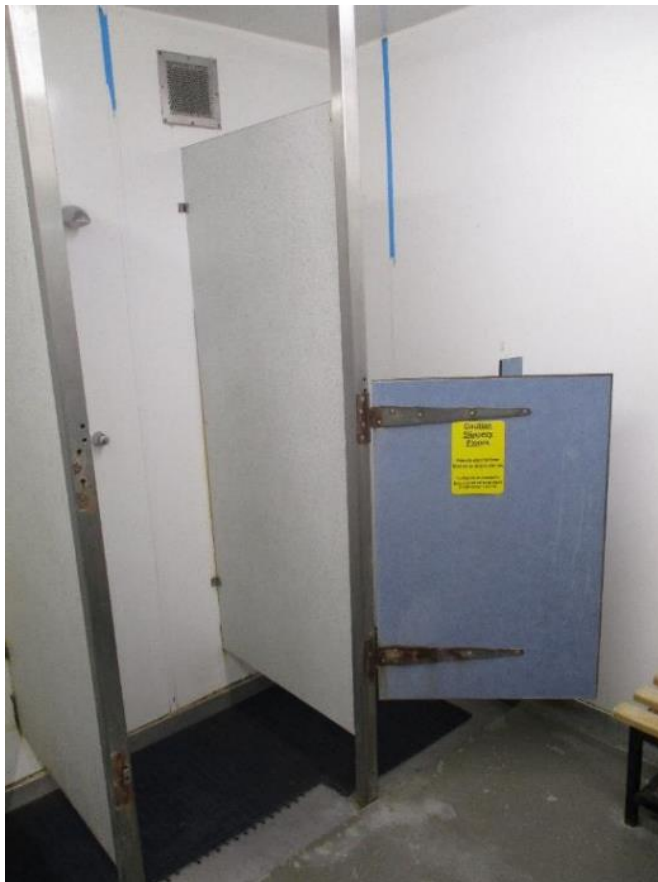
Broken shower doors on Mountbatten unit
