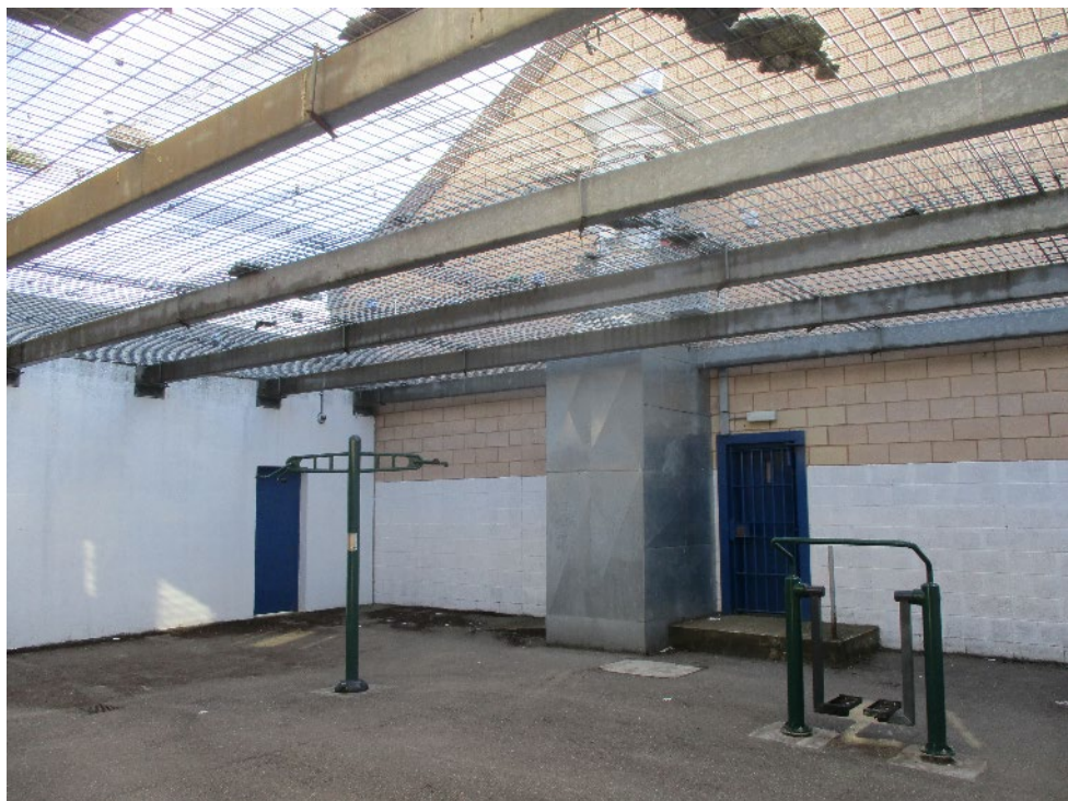
Second segregation unit exercise yard with rubbish on netting
