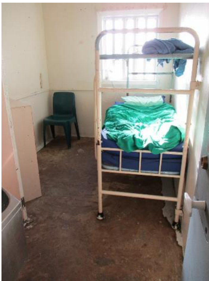
K wing cell with no floor or curtain
