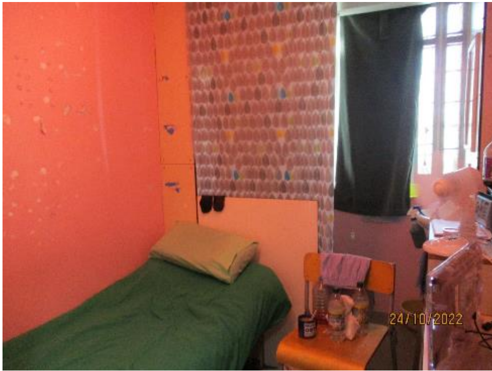
Cell requiring redecoration on residential unit 3
