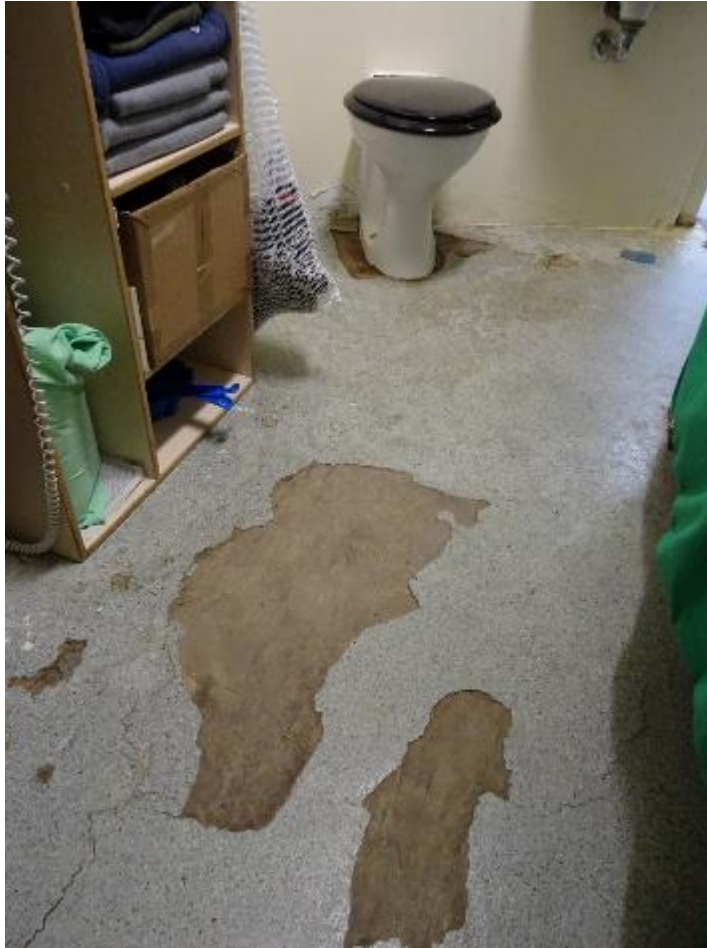
Poor flooring in cell
