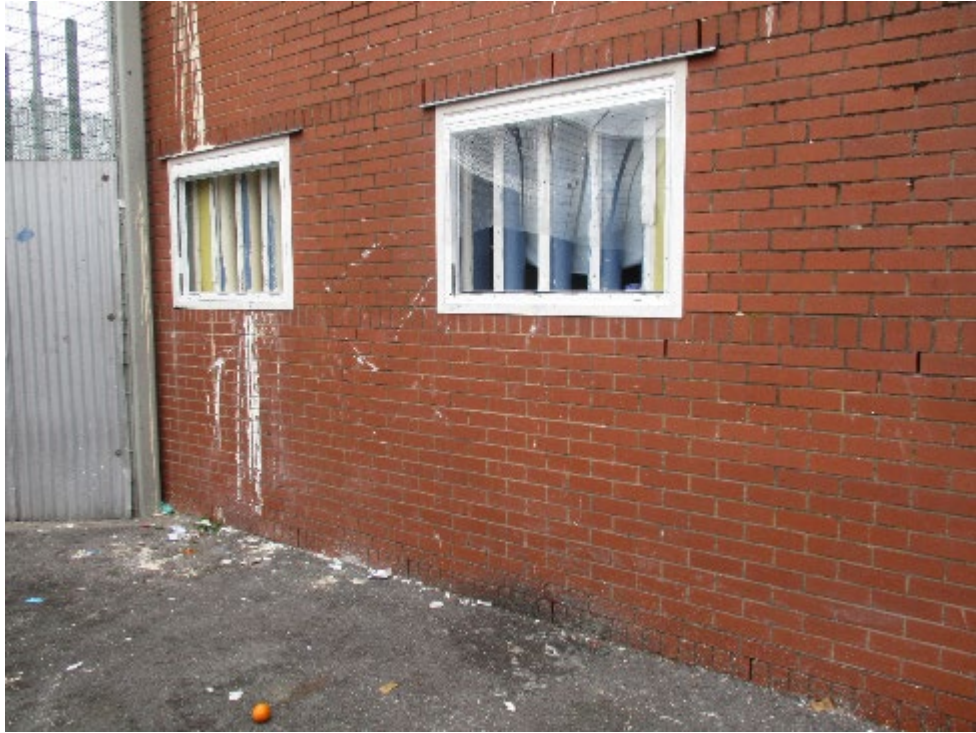
Broken windows on B1
