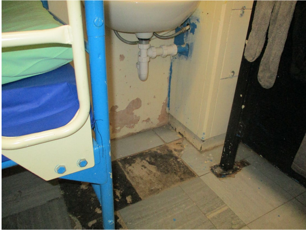
First night cell with damaged flooring
