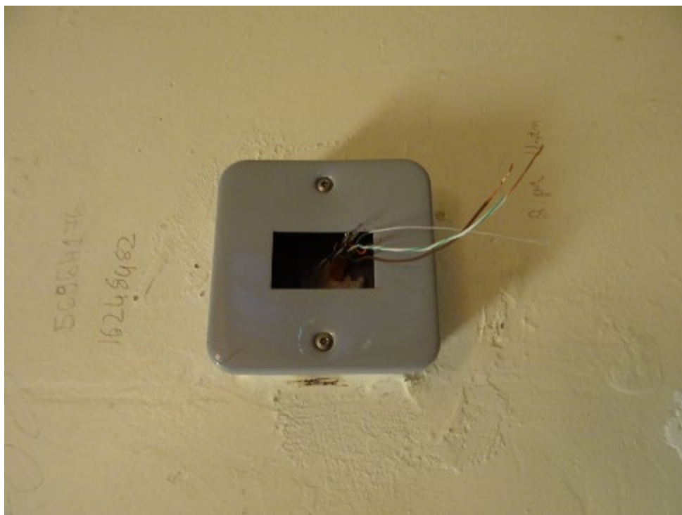
Damaged telephone cabling in cells
