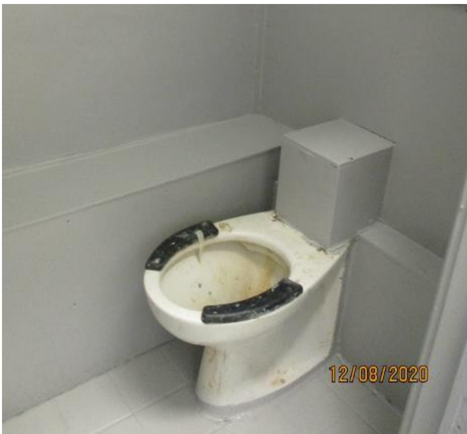
Dirty toilet in reception
