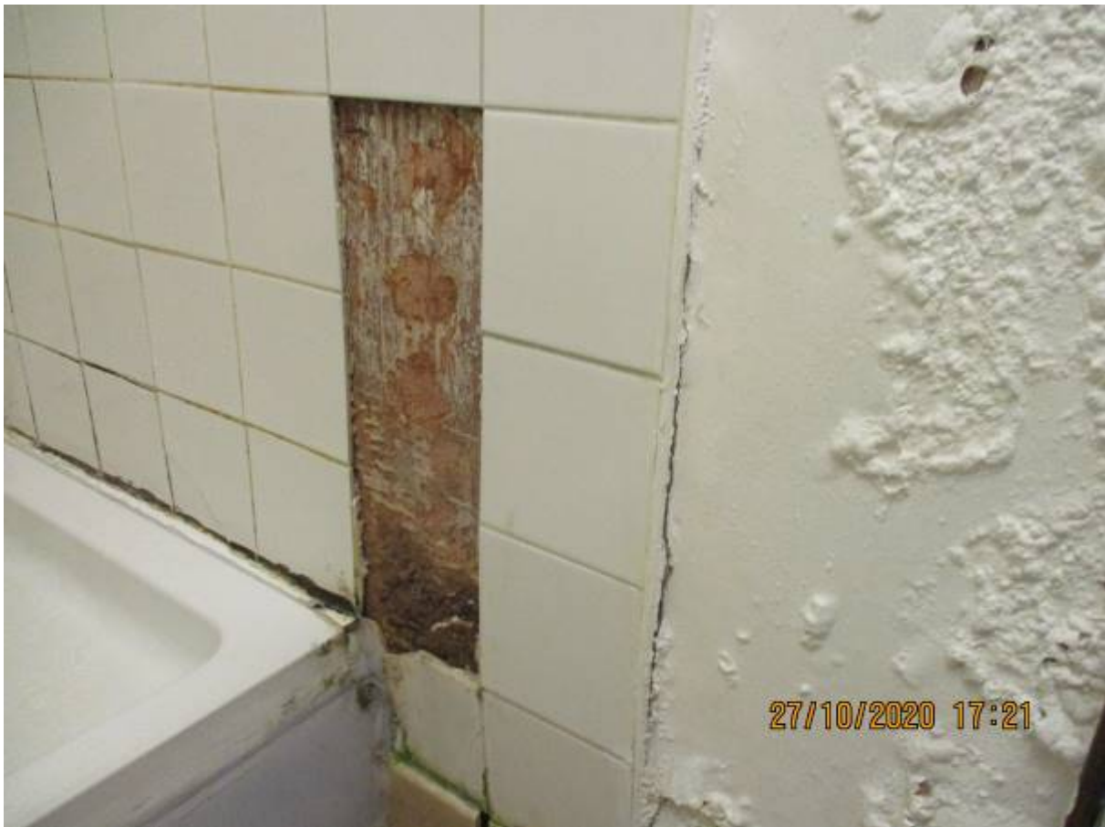
Poor quality shower facilities
