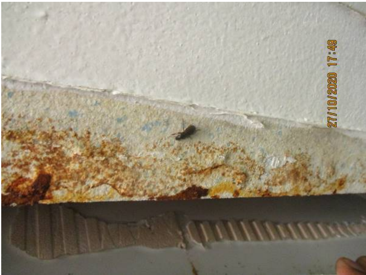
Poor quality shower facilities
