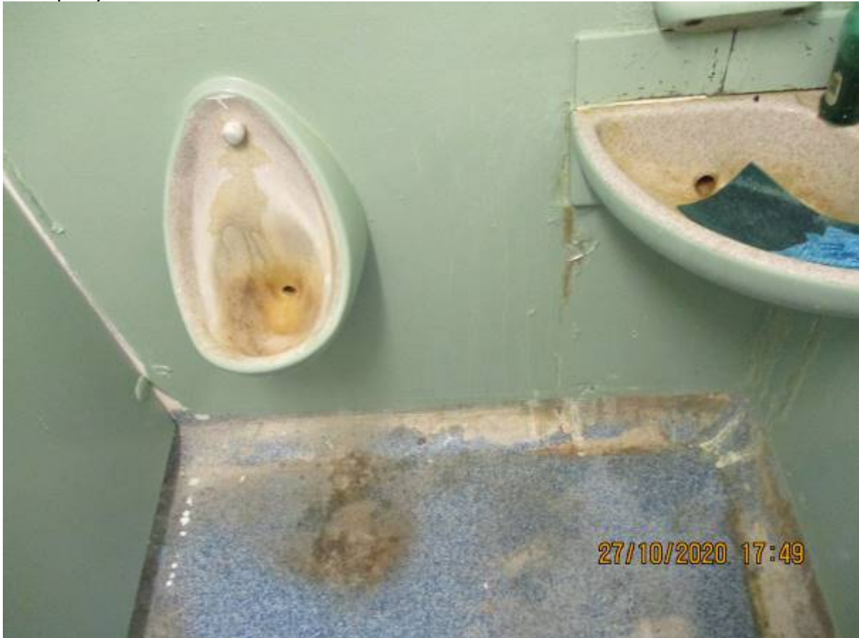
Poor quality bathroom facilities
