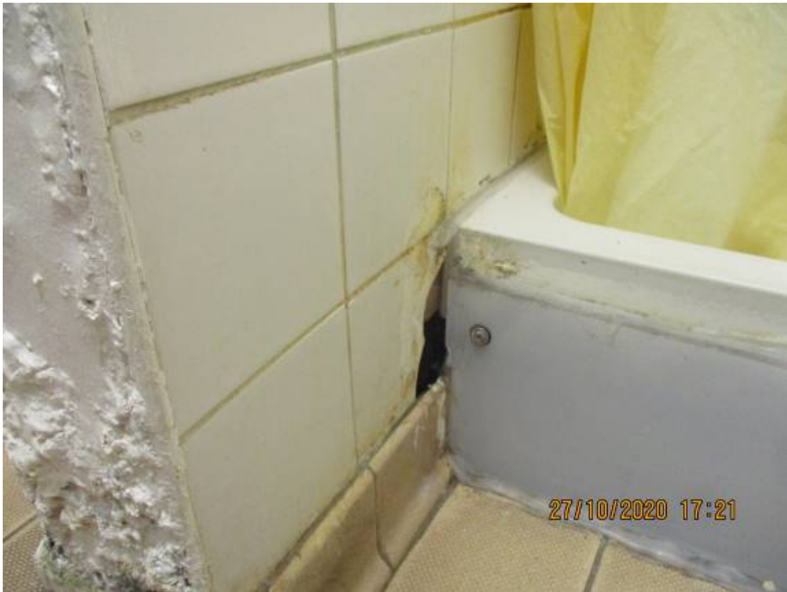
Poor quality shower facilities
