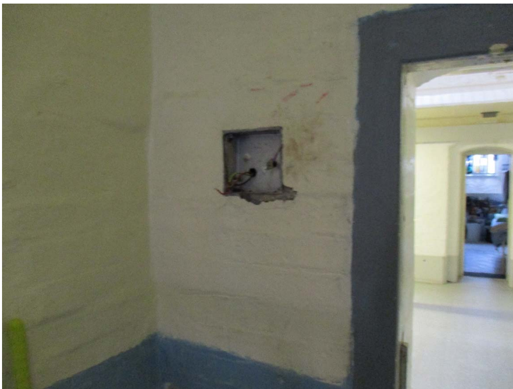
Photograph 6. Occupied cell with exposed live electric wires used by the prisoner to operate the cell lights
