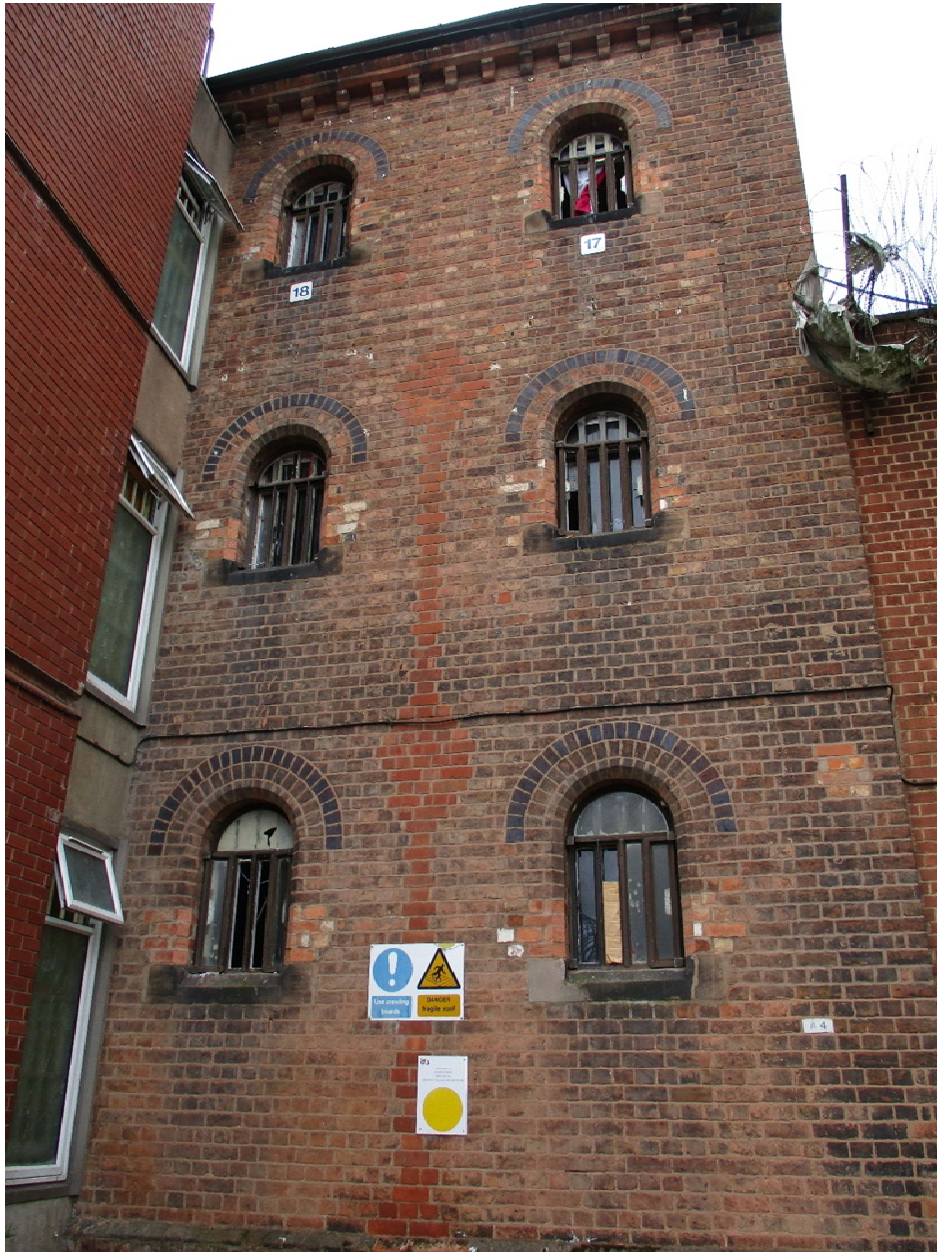
Photograph 2. Broken and missing cell windows
