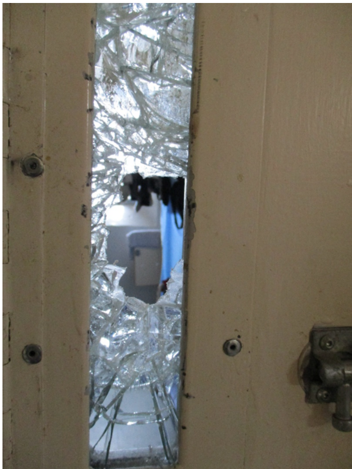
Photograph 4. Broken cell observation panel
