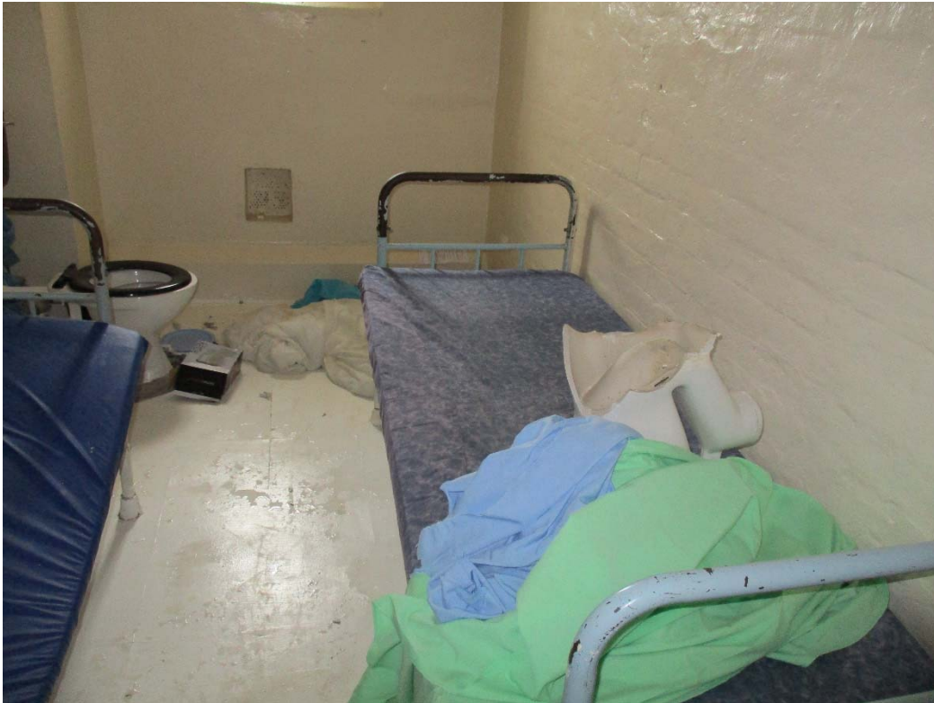
Photograph 1. Flooded and damaged cell
