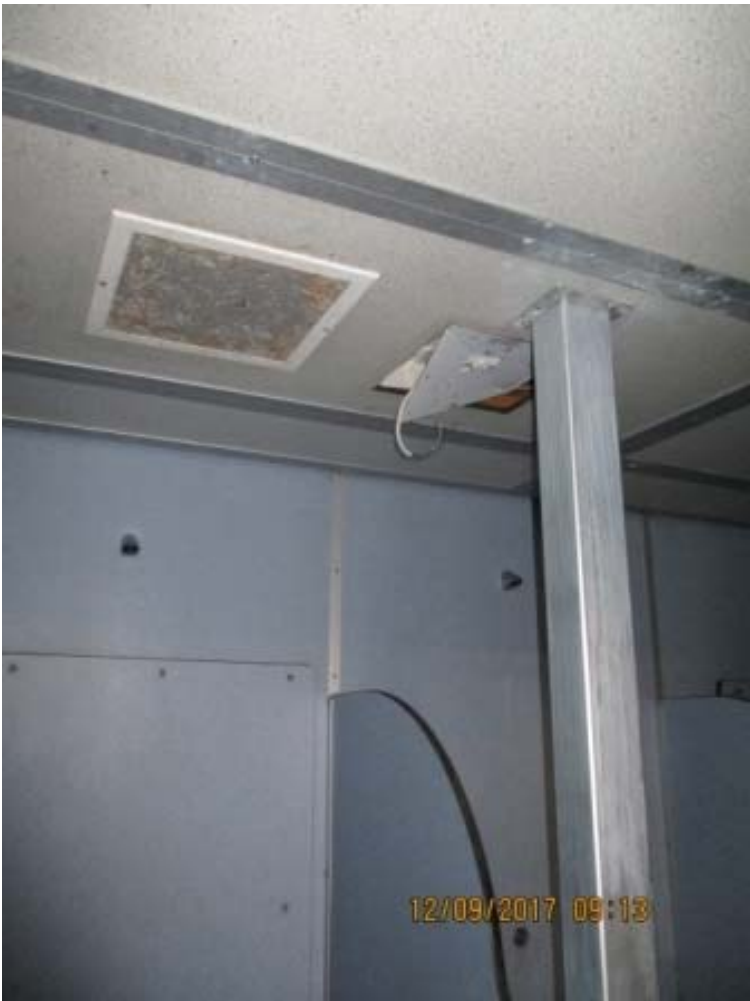
Shower unit with protruding electric cable.
