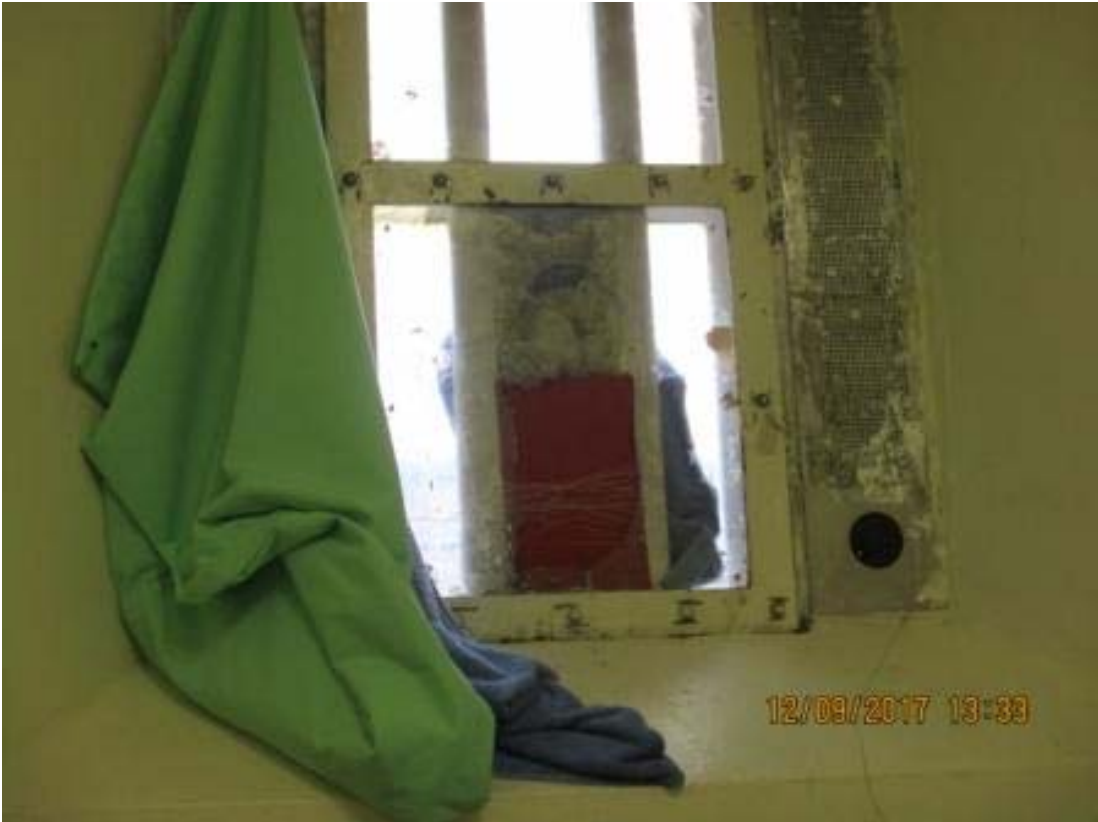
Broken window in a cell.
