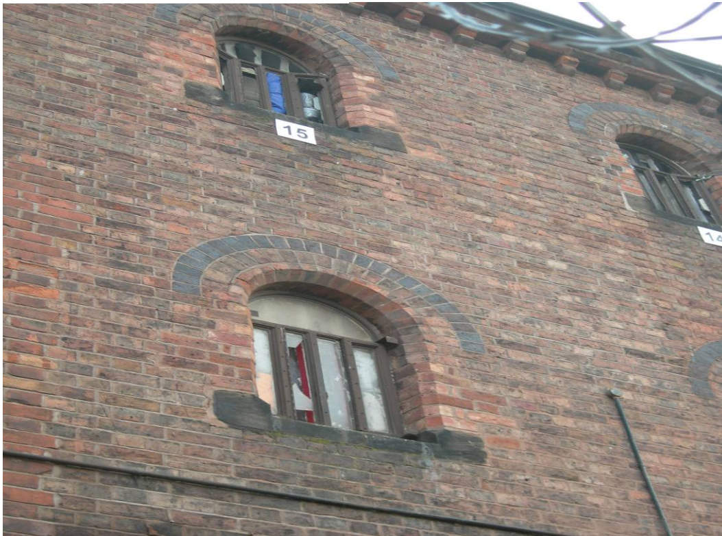
Missing and damaged cell windows
