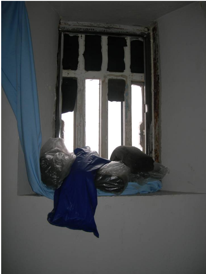
Missing and damaged window in a cell
