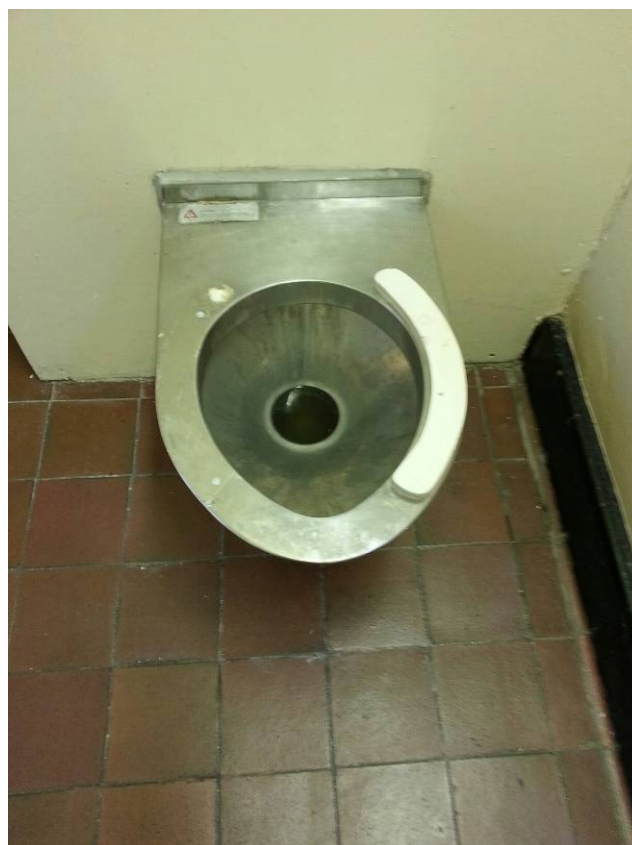
Missing toilet seat, Prestatyn
