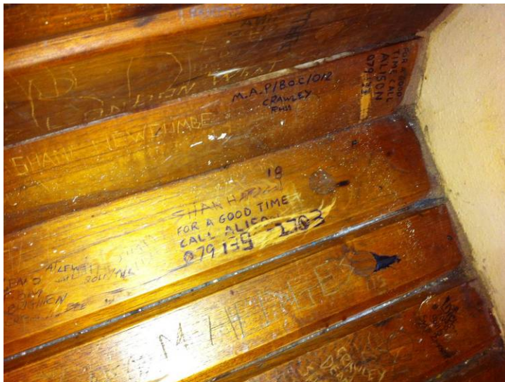
Graffiti on a bench at Lewes Crown Court. The wide spaces between the slats are also potential ligature points
