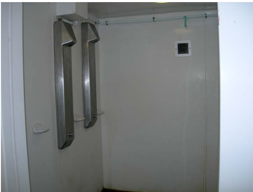
Poor shower units on Sarum unit.
