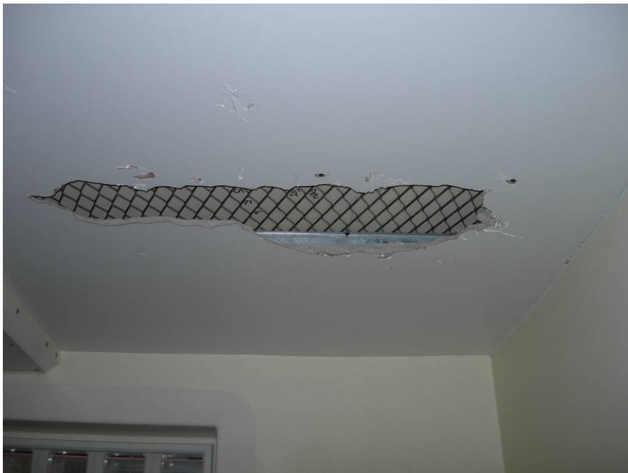
Potential ligature points exposed by damage to the segregation cell ceiling.
