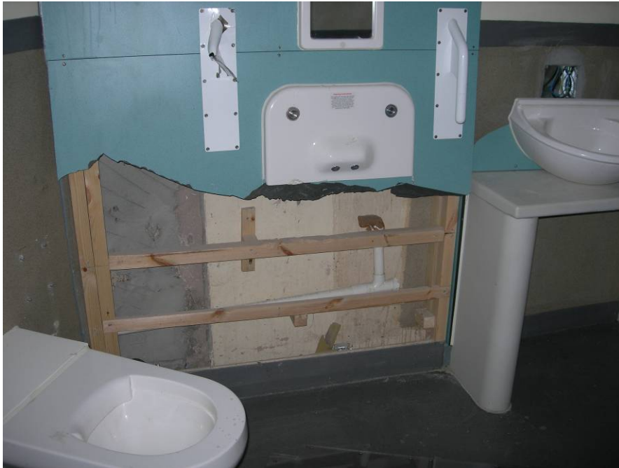
Damage to the fittings and fabric of a segregation cell wall.
