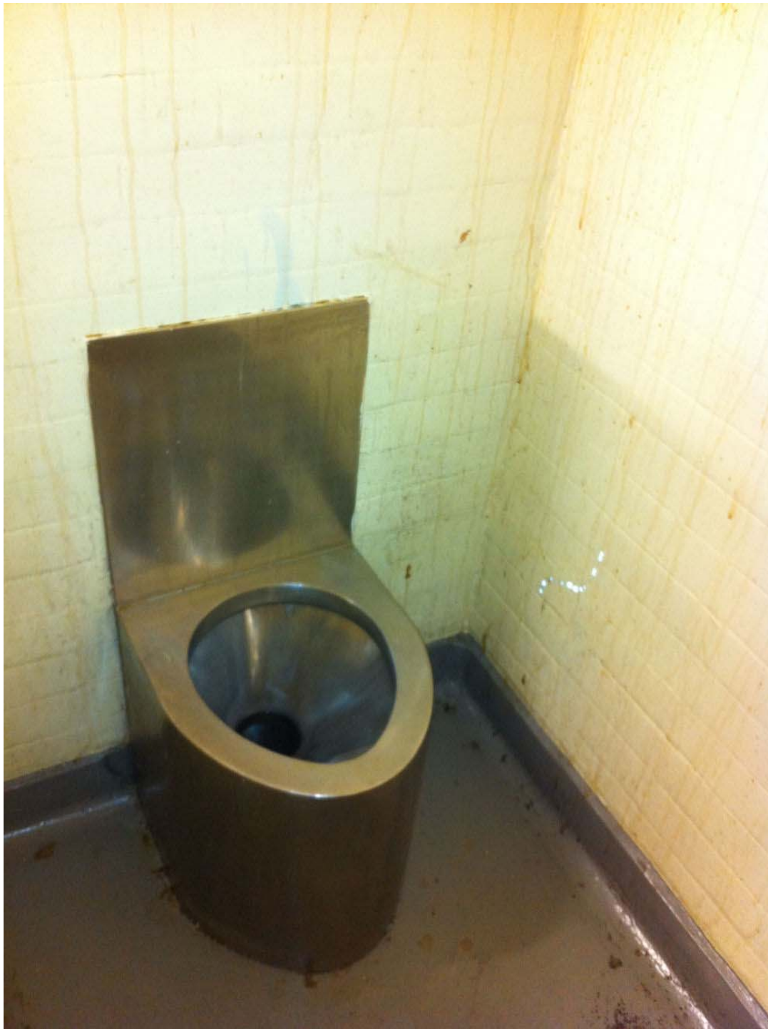
In-cell toilets at Sefton Magistrates' Court with soiled walls and floor
