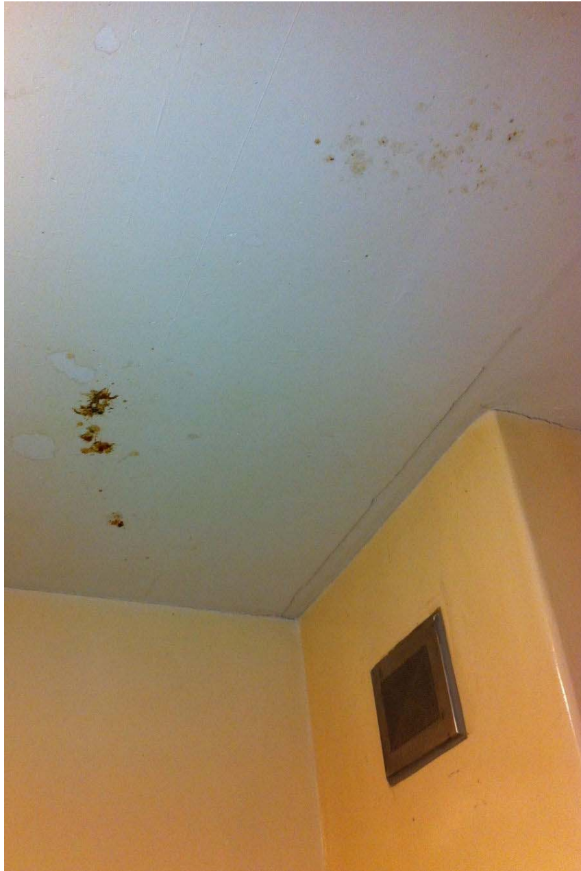
Stained ceilings at St Anne Street
